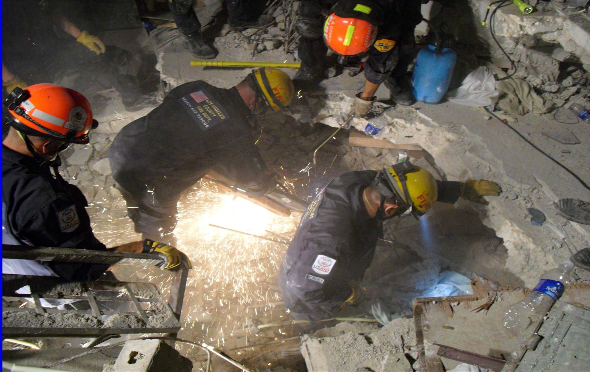
Cutting Rebar with Rescue Saw (Maintain Protector Line or Extinguisher in Place)
